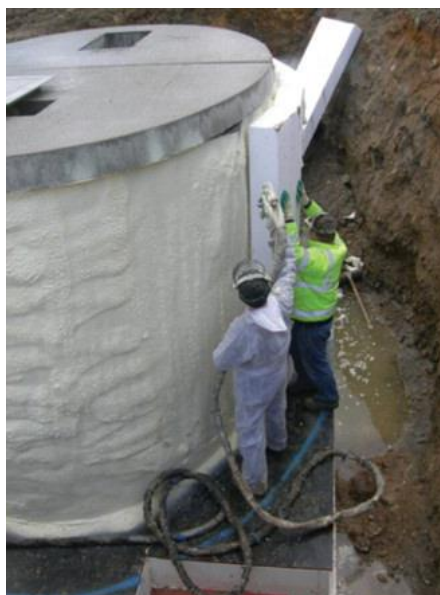
Fig. IV-3. Inter-seasonal storage tank
