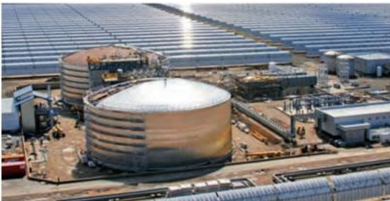
Figure 1.9. Two-tank thermal storage system of Andasol CSP plant [35].
