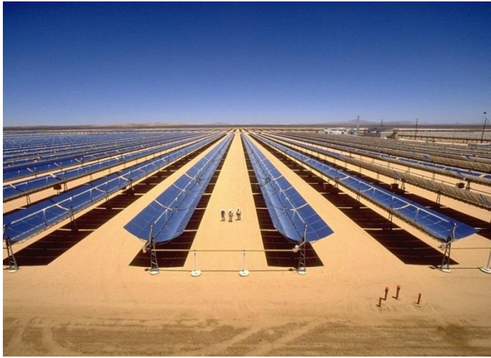
Figure 1.6. Parabolic trough power plant in Mojave Desert [23].
