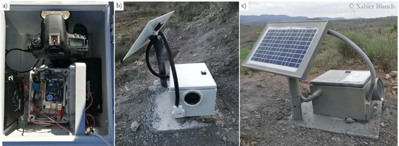
Figure II.19. Photogrammetric system mounted at Puigcercós. a) Internal view of the camera module composed of a camera and the auxiliary control system. b,c) Exterior views of a module: b) Installation works and c) final integration with the environment.
