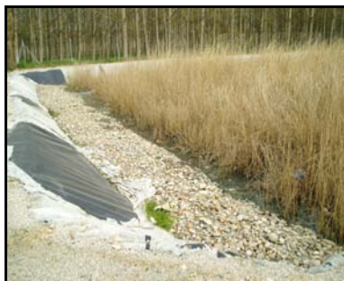
Figure 4.37. Imperfections in the protective waterproofing layer.
