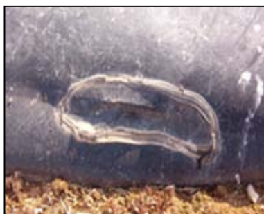
Figure 4.32. Detail of a repaired hole made by rodents in a waterproof membrane.
