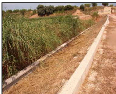
Figure 4.14. HSCW with land-based cell with a concrete pipe at the upper part of the dike.
