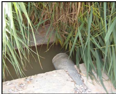
Figure 4.8. An open channel wastewater distribution system.
