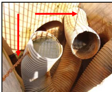
Figure 4.36. The water level controller mechanism flexible tube. The red arrows show the rusty chains which hold the tubes.
