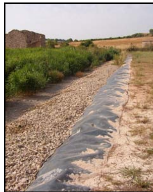
Figure 4.12. Photograph showing the waterproof membrane of an HSCW secured to the upper part of a dike.
