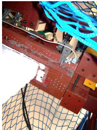
Figure A1. 127 Vertical steel profiles to constrain the horizontal movement of the distribution beam and screws placed in the hinge plate to grab the upper heading tool
