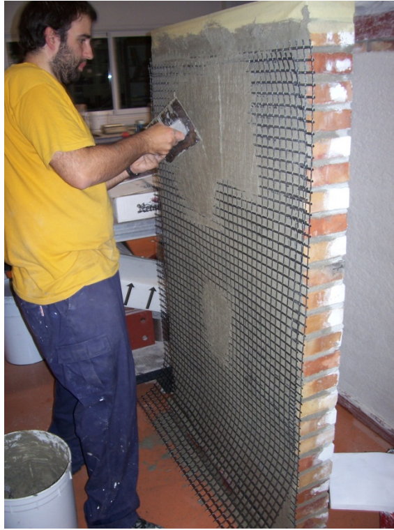
Figure A1. 85 Spreading the second mortar layer of a two grids TRM strengthening (wall W#26)
