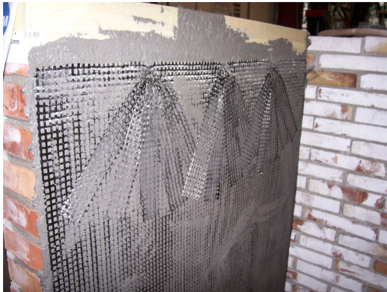
Figure A1. 84 Wall W#28 with the fibre grid and the connectors embedded into the first mortar layer.
