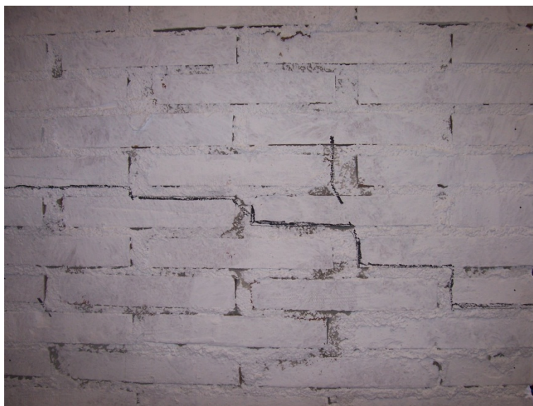
Figure A1. 162 Initial crack at the tensile side of the wall W#14 before testing
