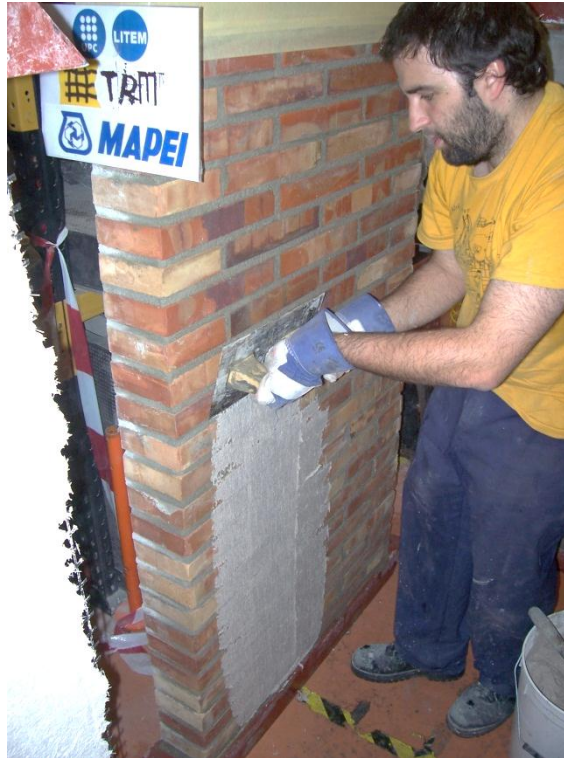
Figure A1. 81 First layer of Planitop HDM Restauro mortar. Upper are of the wall covered to prevent the mortar to stack on it.
