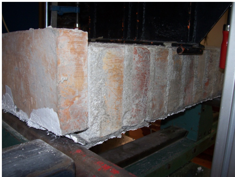
Figure A1. 52 Shear failure of the sample X6. TRM debonding near the support. Masonry joint failure.
