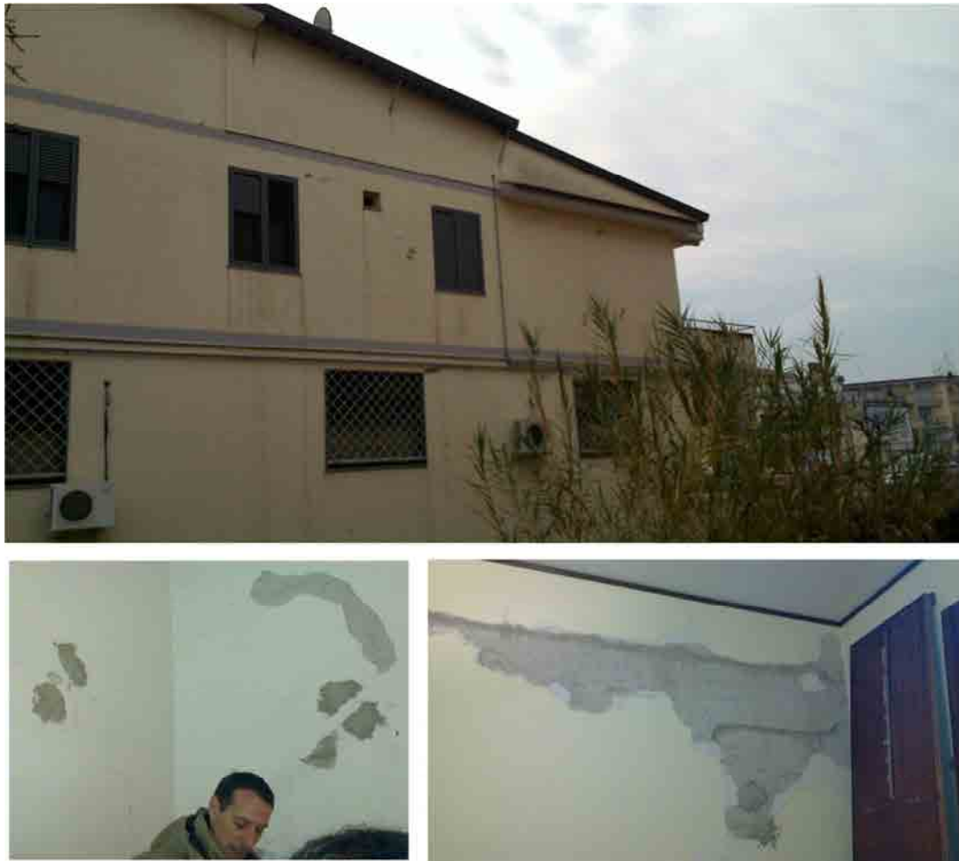
Figure 3.7: example of cracks monitoring in Telese Terme
