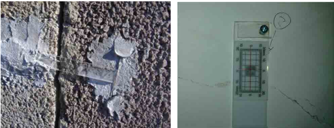
Figure 3.6: glass cracks monitoring system (left); "tell tales" cracks monitoring system in Telesse Terme (right)
