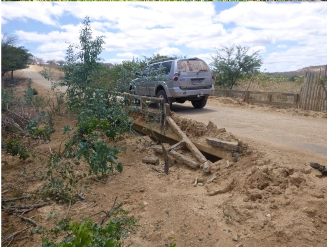
Picture 6. Lower part of the Salitre River Basin – the picture below shows a five meters high bridge on the Salitre river completely silted up.
