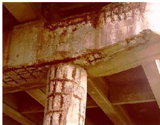
Figure I-1. Structure deterioration due to steel corrosion
