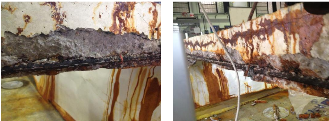
Figure III-31. Final beam state after splitting and spalling
