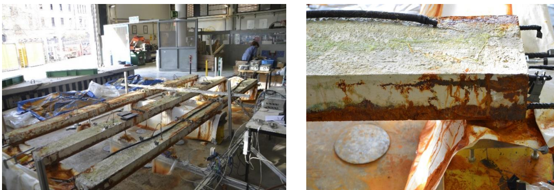
Figure III-8. Final corroded beams aspect. Group 1
