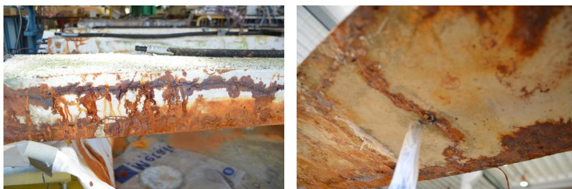
Figure III-24. Damage before testing. Longitudinal and transverse crack
