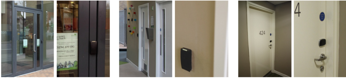
Pictures of the three kinds of ID access filters that we can find in the building. The two pictures on the left show the main building entrance filter. The two pictures in the centre show the lift room filter. And the two pictures on the right show the studio/room filter.
