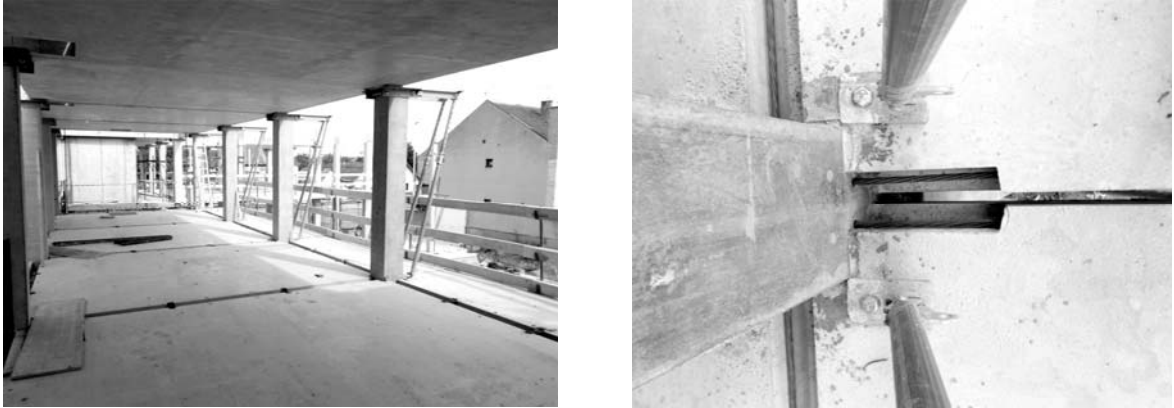
Figure 64: Column-slab joint in IMS Building Technology. Top-view of the standard floor slabs to the left and cantilevers to the right (Petrović & Milovanović, 2012)
