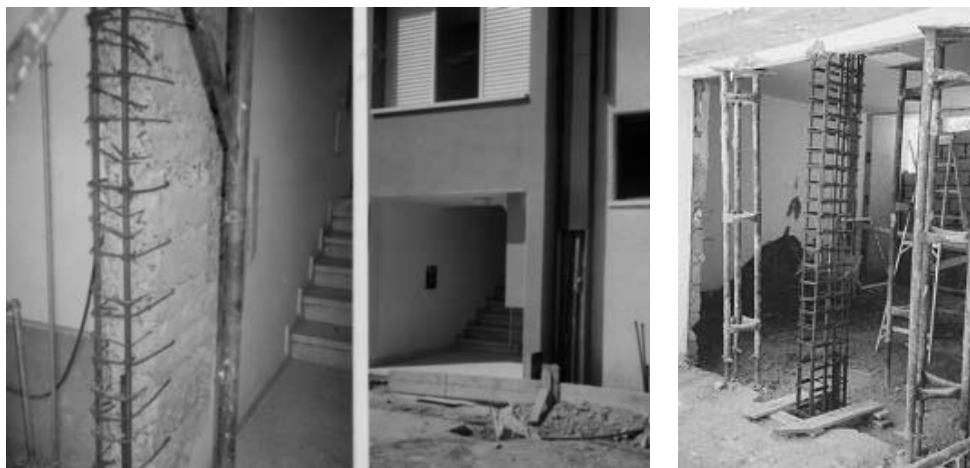
Figure 10: Reinforcement of an inside column (left), adding of a new column (right)
