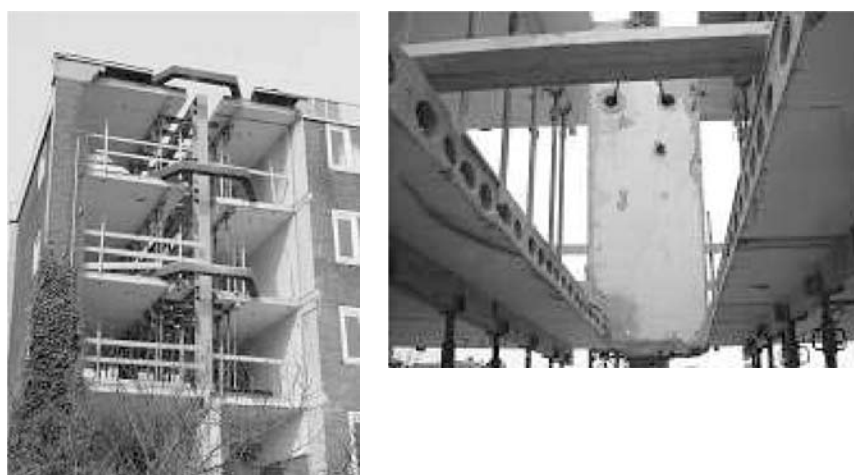
Figure 14: Positioning and connecting of rigid steel frame (left); Removing the bearing wall (right)
