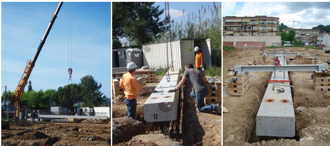
Figure 126 and 127. Placement of precast semi-beams over trenches. Figure 128. Layout of precast semi-beams in plan and height.
