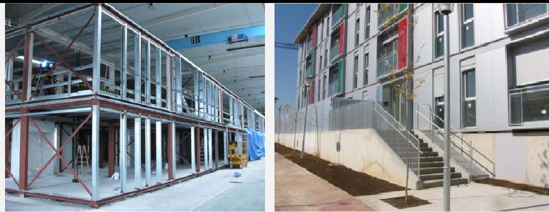
Figure 50. Module system of frames and panels in the factory (A-14). Figure 51. Completed building that uses this system (A-14).
