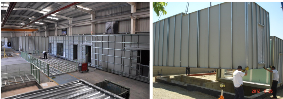
Figure 32. Room modules in a factory (A1-23). Figure 33. Positioning of modules over basement walls. Cladding and the roof then need to be added (A1-23).
