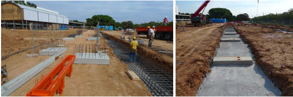
Figure 131. Precast pads, mechanisms for laying out precast pads, and ground beam trench with steel reinforcement inside. Figure 132. Precast pads and cast-in-place ground beam.
