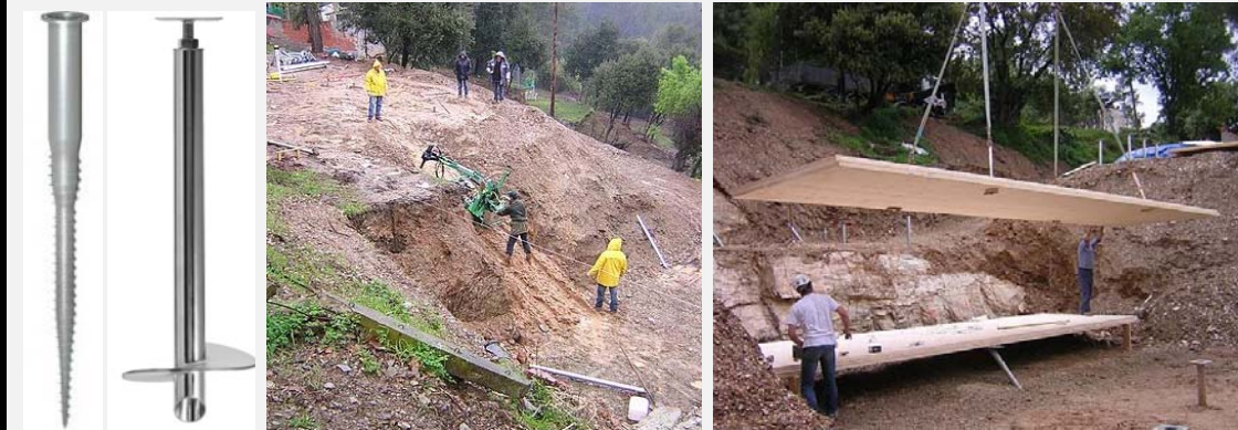
Figures 71 & 72. Screw piles or helical piles. http://blog.business-model-innovation.com/wp-content/uploads/2009/03/358_bild-135x300.jpg http://postechnorthern.ca/wp-content/uploads/2014/07/pic_pile.jpg Figure 73. This machinery could be suitable for cramped and limited-access conditions. Figure 74. Piles can be driven either vertically or at various angles of inclination to increase the support on lateral loads.
