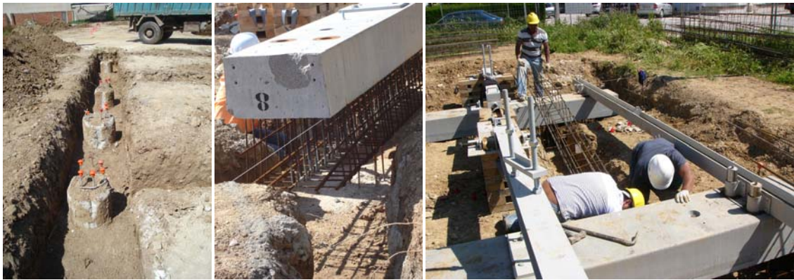
Figure 116. Continuous flight auger piles. Pile heads were demolished and rebars were protected. Figure 117. Placing the semi-prefabricated ground beam over the piles with a crane. Figure 118. Placing reinforcing rebars of tie beams inside trenches.
