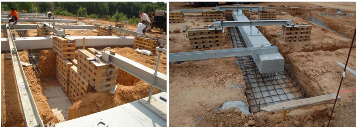
Figures 109 and 110. As shown in the images, the semi-prefabricated beams could be adapted to the different depths of the soil with good bearing capacity (A1-15) (Appendix 1).
