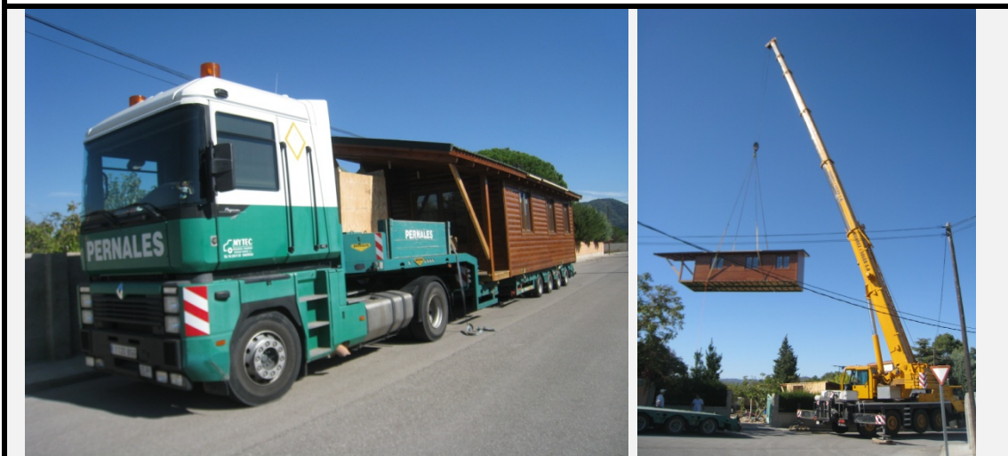
Figure 54. The module is transported to the site on a lorry (A-28). Figure 55. The module is placed on the plot using a crane (A-28).
