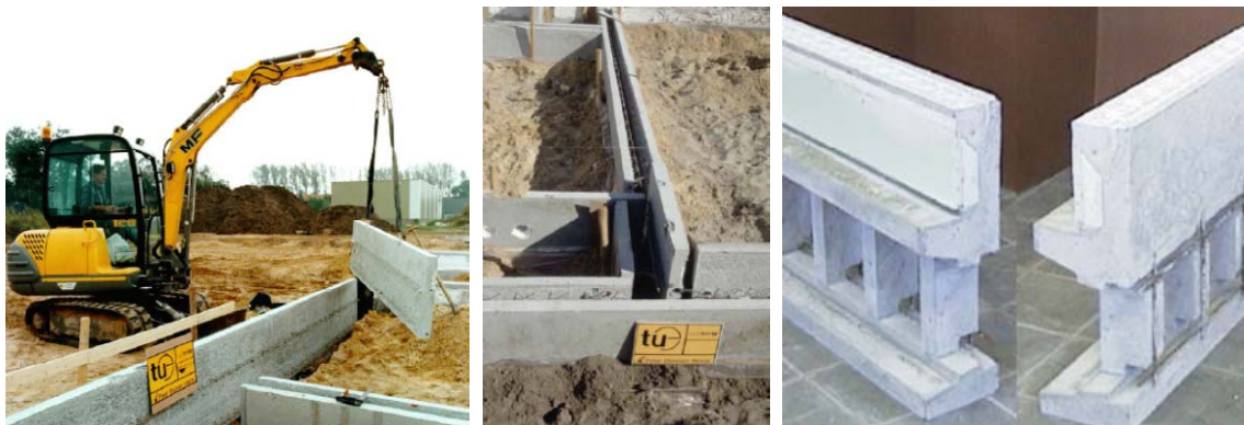
Figures 23, 24 and 25. Faas Moonen designed an accurate foundation to avoid potential dimensional tolerance problems between the foundation and the industrialized dwelling [Moonen, 2001, p. 3.34 & 3.45].
