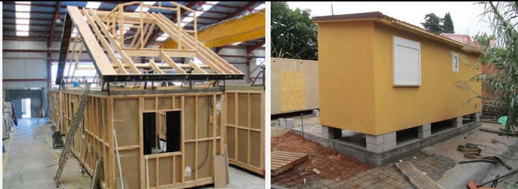
Figure 52. Construction of a module in the factory. It is comprised of frames made from a combination of steel and timber. Figure 53. The module positioned on-site. Windows and doors are sealed with shutters or with particle board to prevent damage in transport and handling (A-27).
