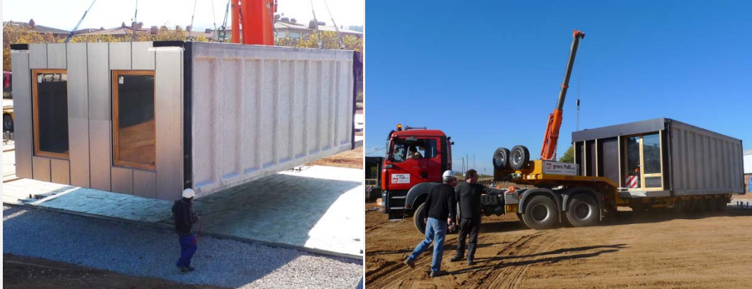
Figure 38. The walls are impregnated with fire retardant foam (A1-16). Figure 39. The modules required special transport (A-16).
