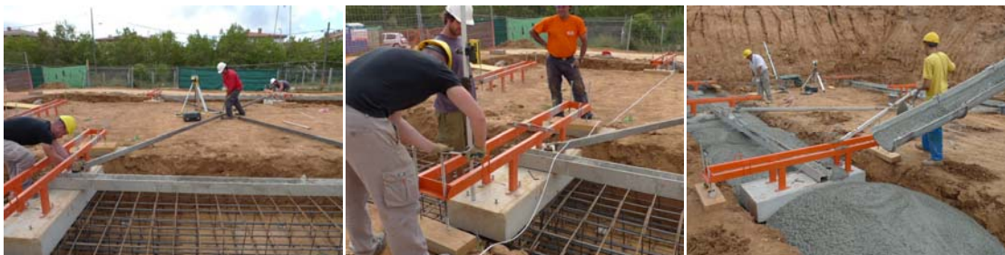
Figures 133, 134 & 135. It was laborious to position precast pads in the A1-16 case study. They were set out along the ground beam, in diagonal and in height.
