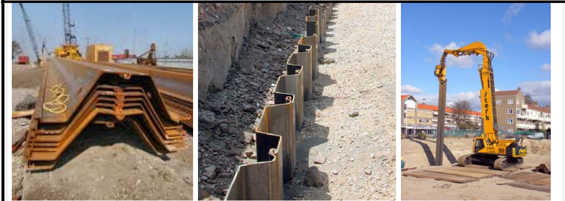
Figure 85. Storage of sheet piles. http://naavaay.com/wp-content/uploads/2012/10/Sheet_pile_New_Orleans-09-04-05.jpg Figure 86. Installation of sheet piles. http://www.imeco.at/pro/sho/img/sho0604.b.jpg Figure 87. Removal of sheet piles. https://upload.wikimedia.org/wikipedia/commons/7/7d/Etec_880_special_removing_Sheet_pile_walls_(1).jpg
