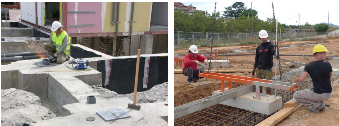
Figure 5. The connectors were cut off using an angle grinder, because they were not positioned in exactly the right place (A1-14). Figure 6. Prefabricated pads were positioned over the foundations that had been constructed on-site. These prefabricated pads had the connectors set in place in the factory (A1-16).
