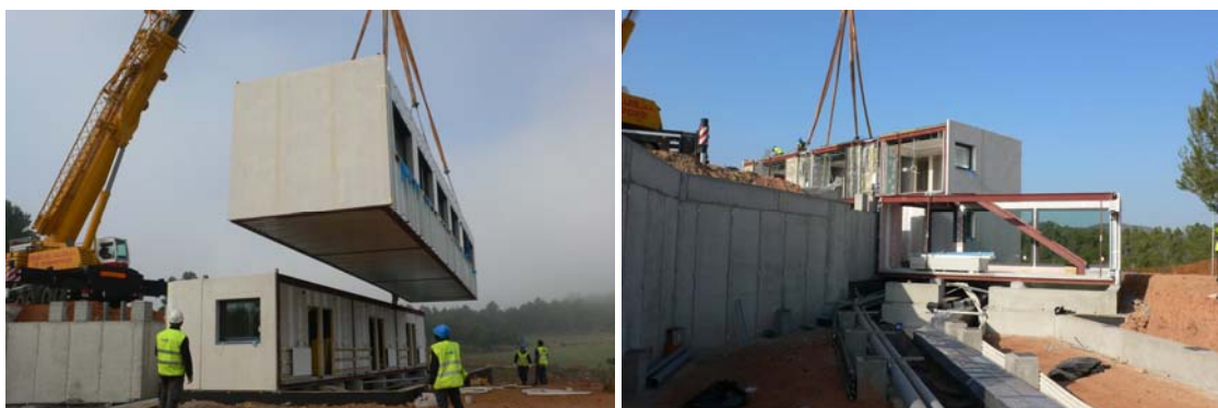
Figures 112 and 113. In A1-13 (Appendix 1) the modules had to be placed over the foundations in two steps. In the first step, the module was rested on the foundations. In the second step, it was positioned in its exact place.
