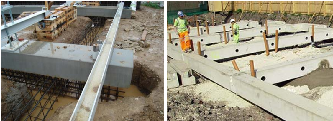
Figure 122. Cast-in-place tie beams are below the level of prefabricated semi-beams. Figure 123. In a prefabricated foundation system, the prefabricated tie beams can be at the same level as the precast ground beams.
