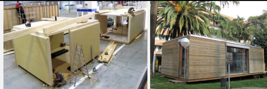
Figure 46. This is a modular system of wood with panel walls (A-6). https://www.youtube.com/watch?v=npTcxWIDbsQ Figure 47. The module positioned on-site (A-6).
