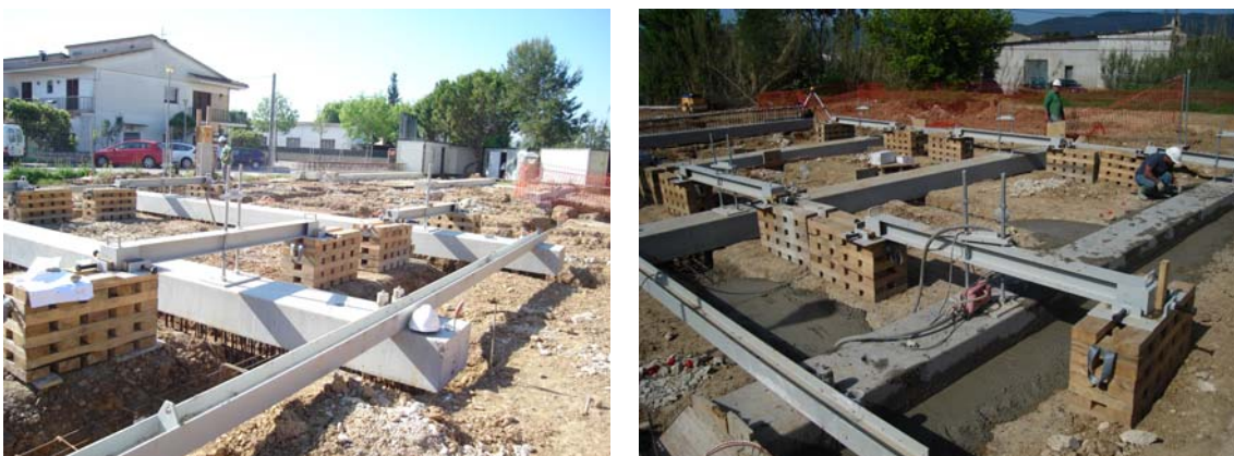
Figure 119. Precast semi-beams laid out in plan and height. Figure 120. Tie beams and the lower parts of ground beams were concreted.
