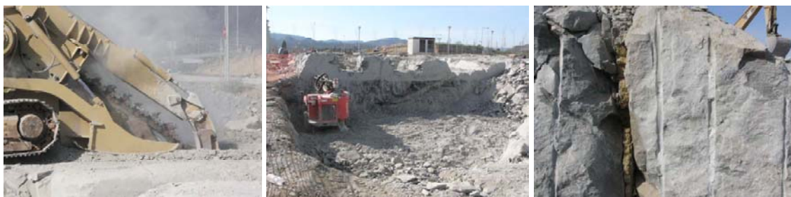
Figure 142. Cat excavator digging a trench. Figure 143. Boring machine boring holes in the ground to inject expansive mortar to break up the rock. Figure 144. Bore holes with the remains of expansive mortar.
