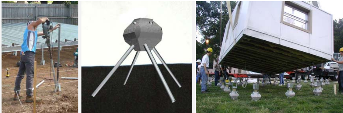
Figure 82. A driving hammer is required to install this type of micropiles. https://greentasreno.files.wordpress.com/2010/04/installing-mega-anchors-4.jpg Figure 83. Caps can be made of steel or concrete http://diamondpier.com/ Figure 84. Installing a room module over a group of micropile foundation. http://diamondpier.com/
