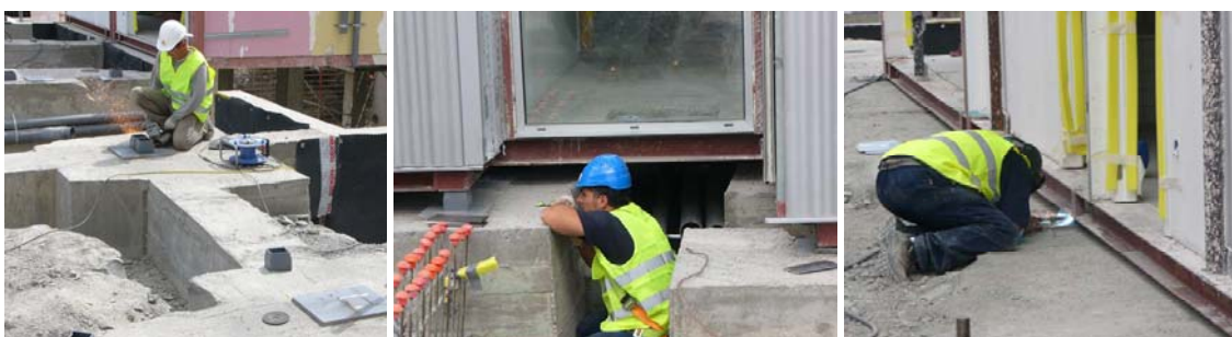
Figure 149. Cutting diverted connectors with an angle grinder. Figure 150. Placement of modules over connectors. Figure 151. Provisionally, the modules were welded over the connectors.
