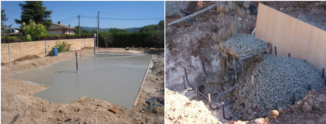
Figures 3 & 4. These are some of the foundations that are constructed for room module buildings. Figure 3 shows a ground slab constructed on-site. Figure 4 illustrates an isolated footing [Jiménez, 2010], which was also built on-site.
