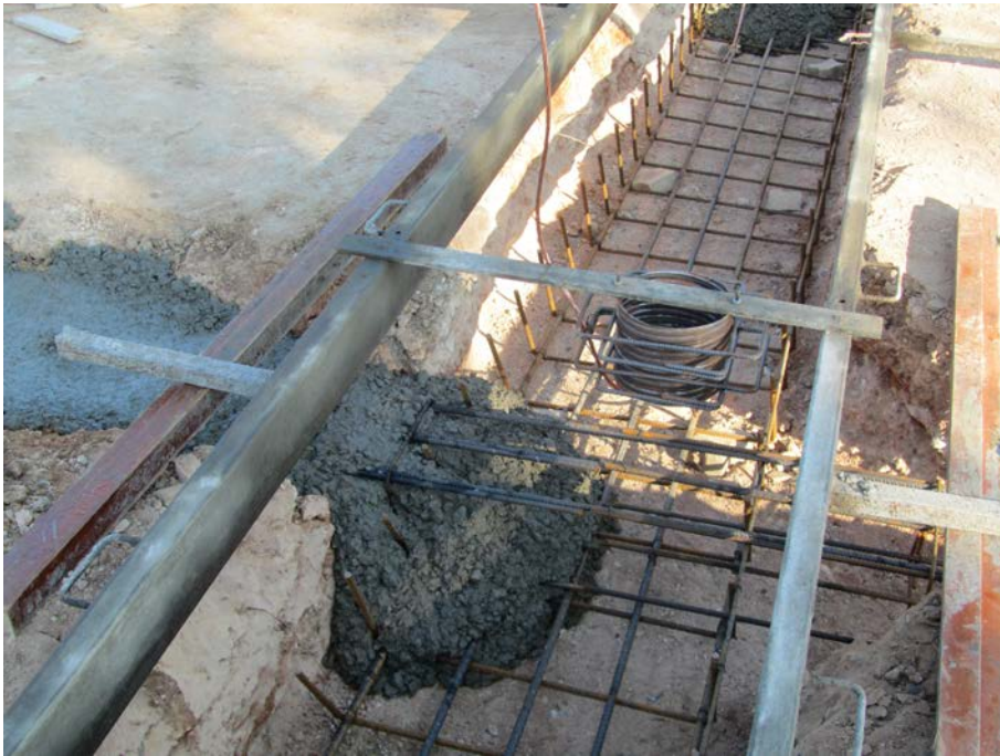
Figure 4. Metal template to position metal cylinders inside strip footings. Once the foundation was concreted, module connectors were placed inside holes.
