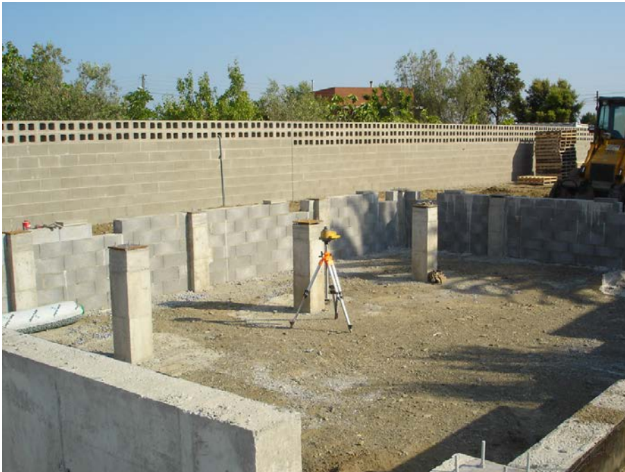
Figure 4. Modules are placed over metal plates, placed over concrete block walls and pillars.
