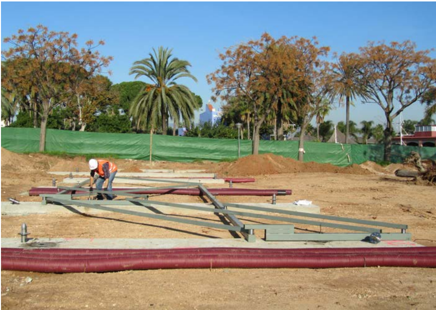
Figure 5. This mechanism set out the location of six connectors at one time.
