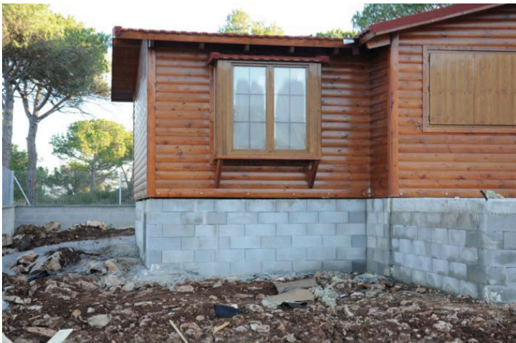
Figure 4. Modules are placed over concrete block walls to form the suspended floor.
