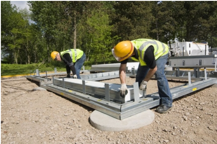
Figures 1. It is not always necessary to build caps. The floor is mounted over precast pile caps. 4
