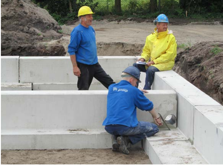
Figure 1. Joints are sealed with mortar. Tie beams have already holes for pipes.
