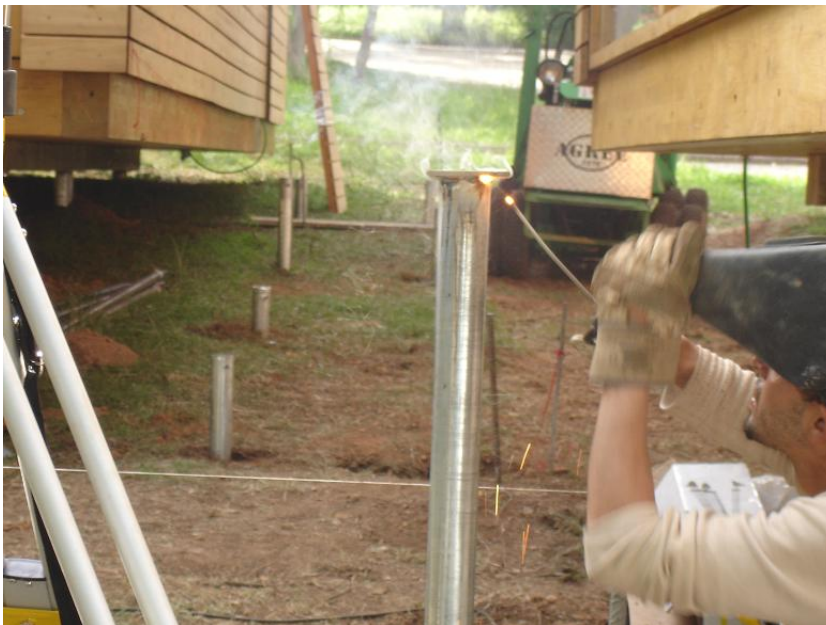
Figure 4. A metal plate was welded at the top of a screw pile.
