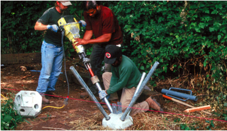
Figure 1. The bearing micropiles must be slid through the holes in the pier, and driven into the soil with an auto driving hammer. 2
