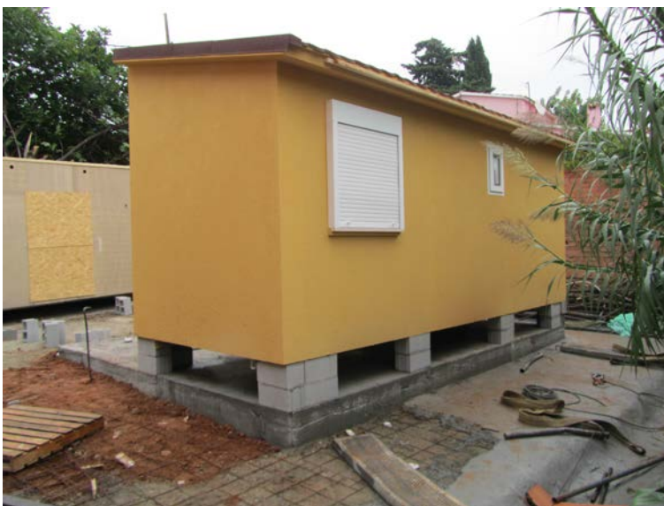
Figure 4. Half house is placed in the right position. It rests on concrete blocks.
