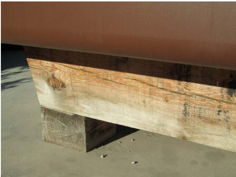
Figure 4. Timber wedges under the timber beams to compensate the slope of the ground slab.
