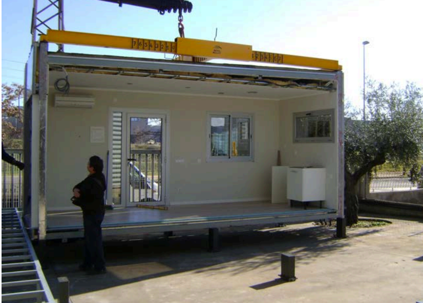
Figure 3. Modules are placed over metal supports. Supports were fixed to the foundation by means rebars and vinyl ester resin.
