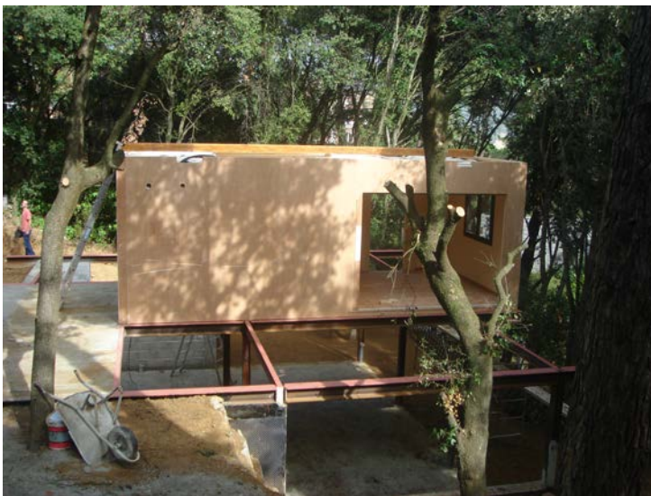
Figure 4. Modules are placed over a metallic structure to take advantage of the slope of the ground and to build the garage under the house.
