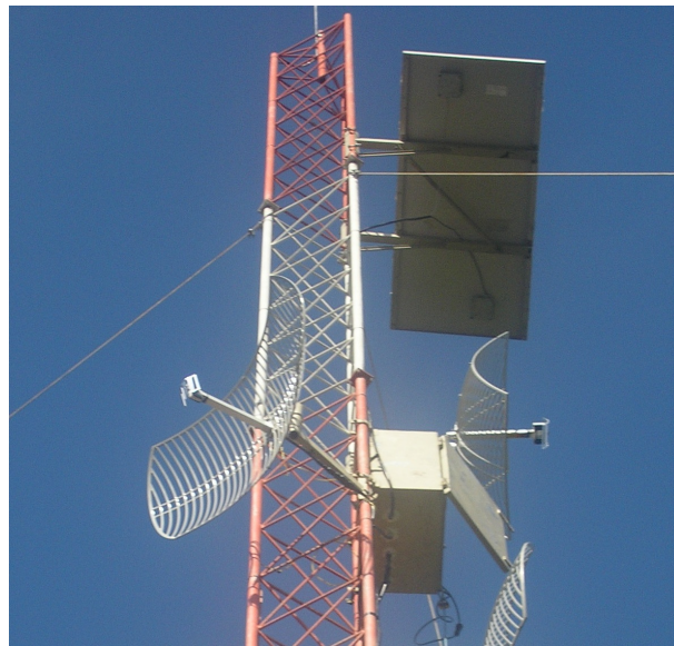
Figure 5.3: Picture showing the real BS, battery, and solar panel employed in the deployment.
