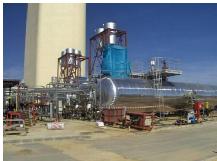
Figure 6. Steam accumulator in solar plant PS10 (Abengoa, Solúcar platform, Seville)
