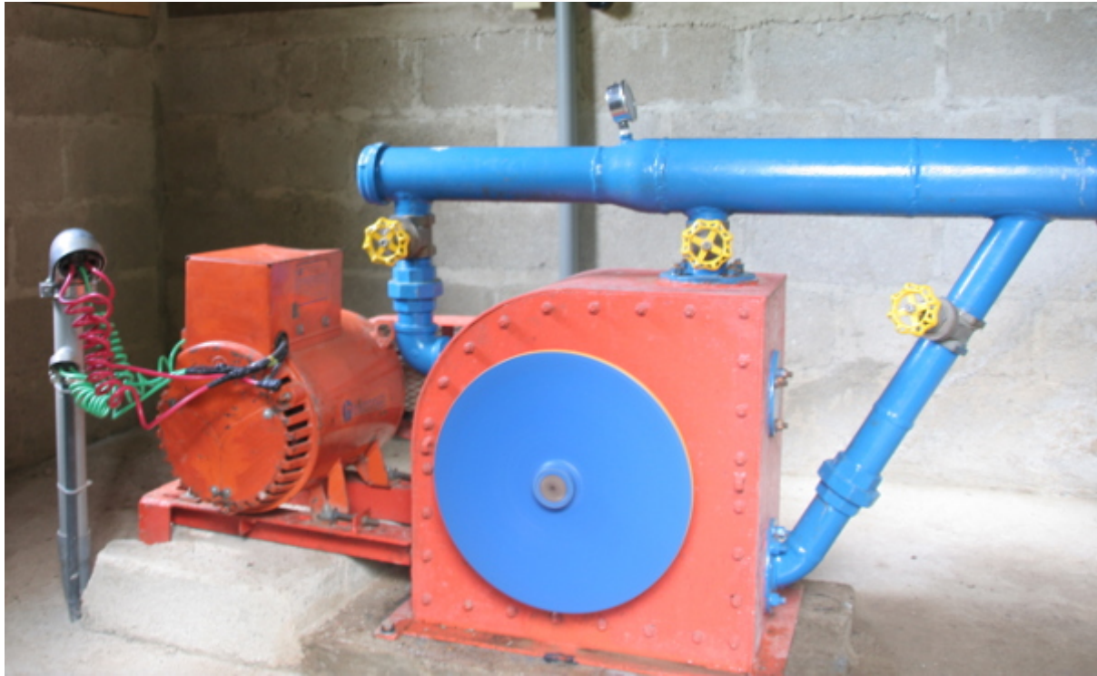
[6.31] Three Jet Pelton Turbine with Flywheel, fabricated and installed in Honduras (author's photo, 2013)
