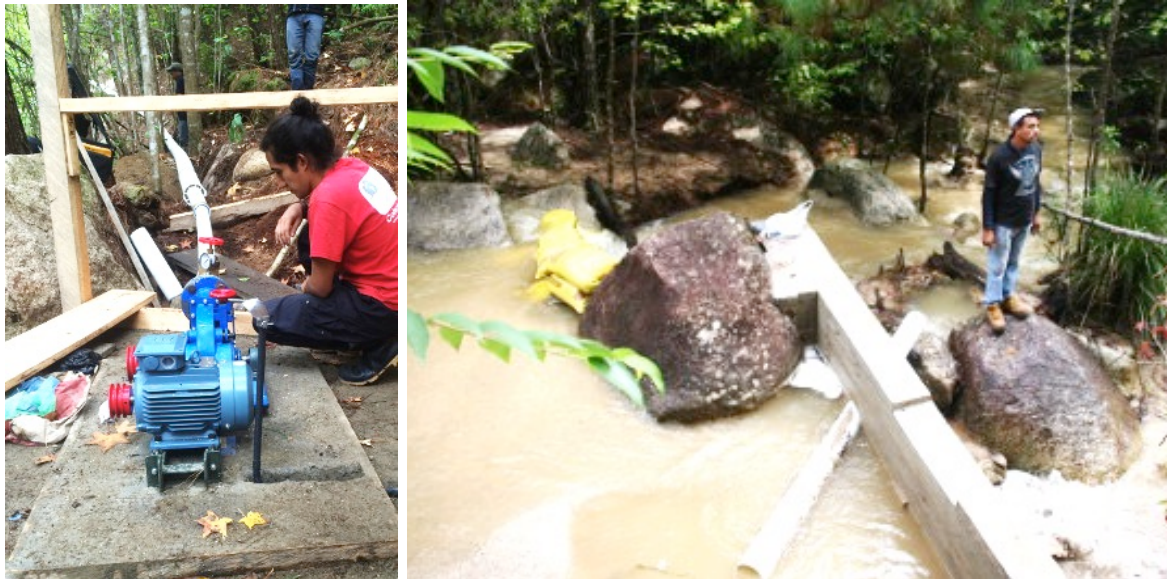
[6.15] Turbine and Generator connected to Penstock (Rodriguez, 2015)
