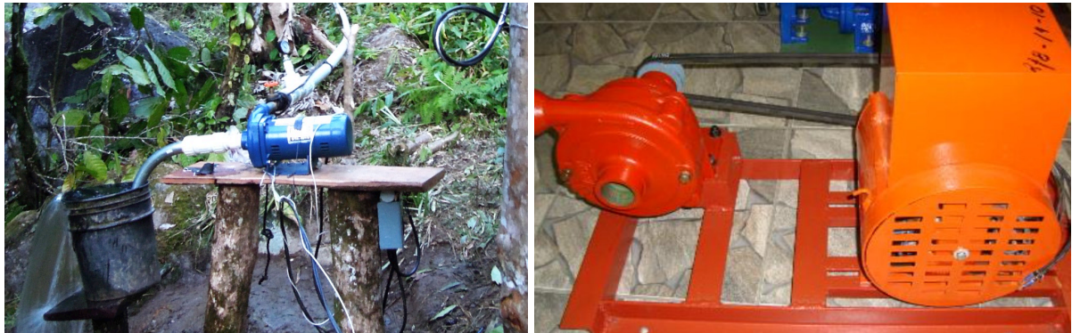
[6.21 / 6.22] PAT Installation in Honduras and PAT with separate Generator, (author's photo, 2012)
