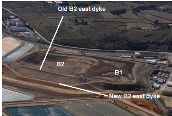
Figure 2.10: Aerial view of the B1 and B2 basins showing the construction of the new B2 east dyke and emplacement of mixture of soil and sludge within the B1/B2 basins, March 2007 (Source: AREVA).
