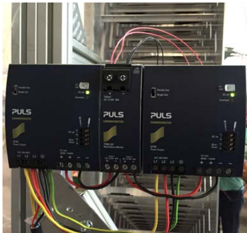
Figure 7.1: Switching mode PSU and redundancy module used in the LST camera.
