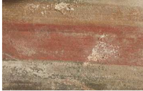
Fig. 4. Pompeian wall painting that presents the degradation phenomena of paints layers
