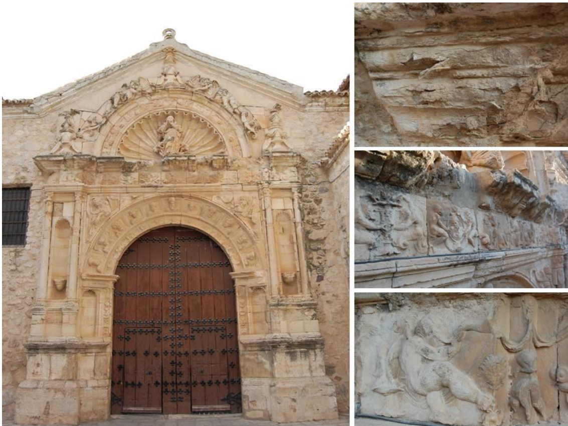
Figure 1. Main portal of the Church of Nuestra Señora de la Asunción (Corral de Almaguer – Toledo) dated mid-16 th century. The pictures show the conservation state of the stone. Material lost, crystallization of salts, physico-chemical alterations by biological agents.
