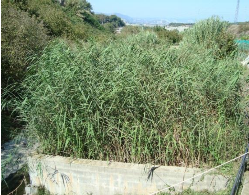
Figure 4.1 STW in Catalonia (Spain). From the top Alpens, Sant Boi de Lluçanès and Seva.
