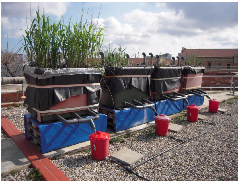
Figure 5.1 Detail of the pilot plant (March 2011)
