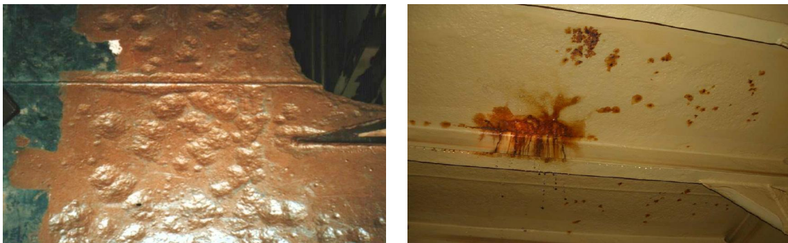
Figure 1.7: Examples of pitting corrosion.
