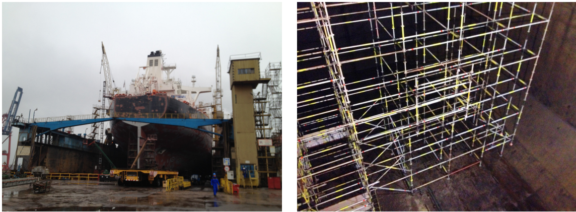
Figure 1.9: Tanker-type vessel prepared for a periodical survey: (left) vessel situated in a dry-dock, (right) scaffoldings installed inside a cargo hold.
