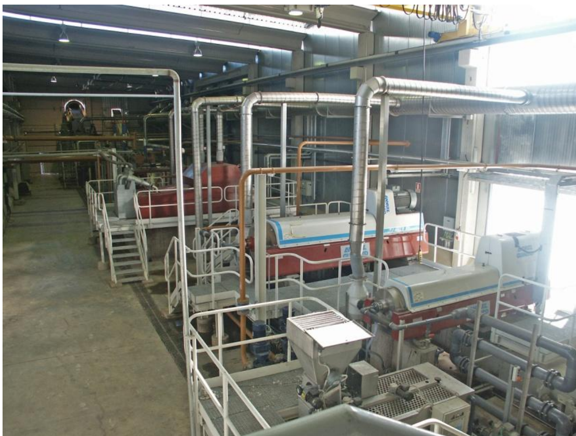
Figure 3.6: Anaerobic digestion area centrifuges
