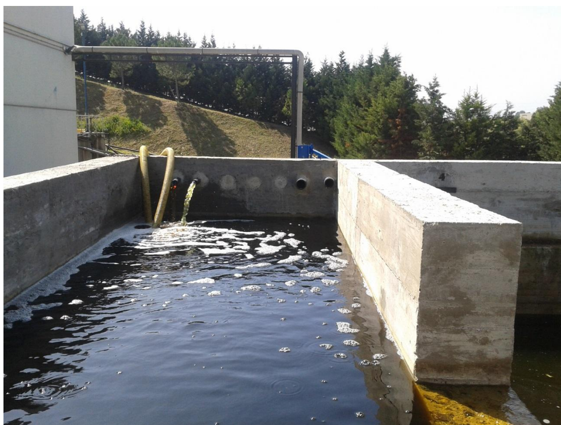
Figure 1.25: Homogenisation tank view 1
