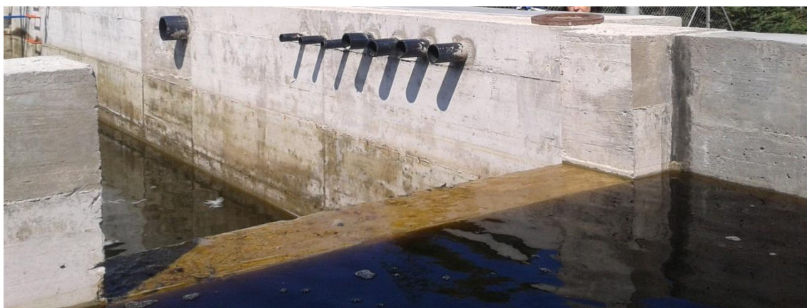
Figure 1.26: Homogenisation tank view 2
