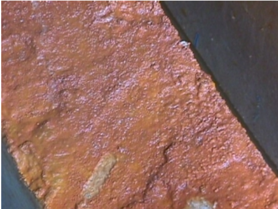
Figure 6.4.16. External face of a SO 4 -attacked beam (plaster formation).
