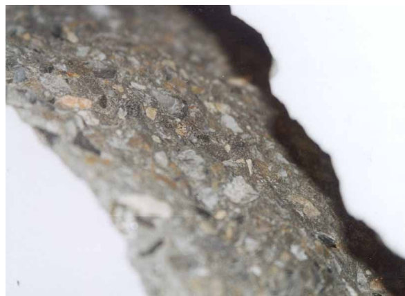
Figure 4.5: Beam specimens without web reinforcement. Crack surface in beam H100/1. Crack goes through aggregates.
