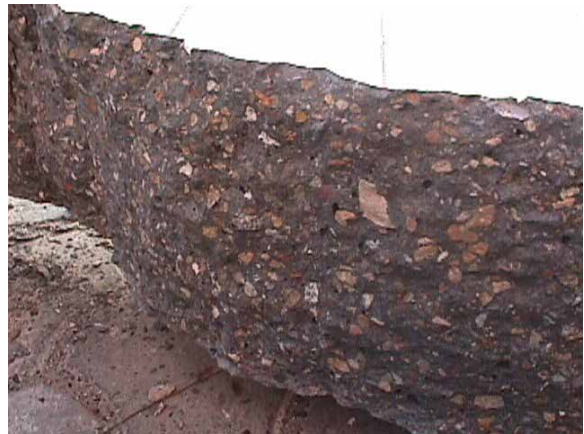
Detail of the crack surface
