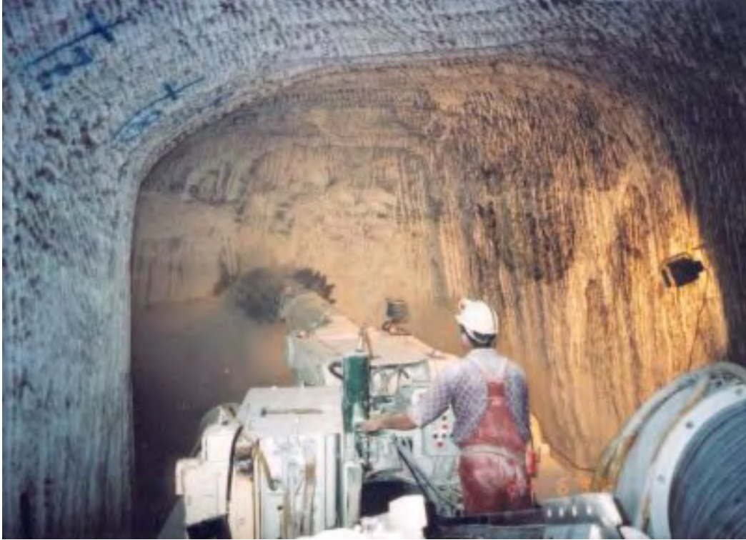
Fig. 2.3 The excavation of a tunnel in salt rock for nuclear waste disposal
