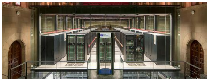
Figure 1.1: Picture of the MareNostrum (MN) supercomputer, hosted inside a chapel.
