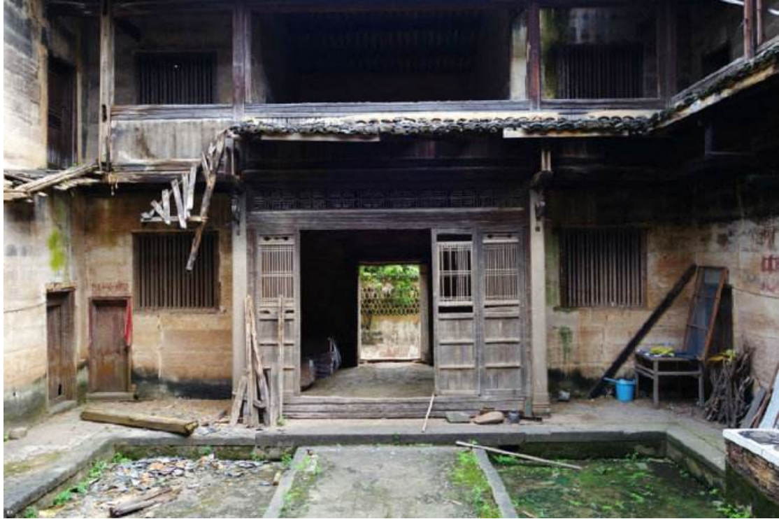
Figure 4-78 Damaged traditional house
