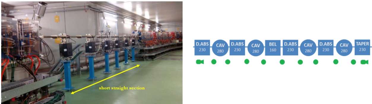
Figure 2-7: Installation location (left) and layout (right) of the 3 rd Harmonic system in the ALBA Storage Ring.
