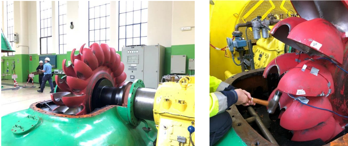
Figure 3.12. Left, view of the turbine with open housing and right, view of impacts in the buckets
