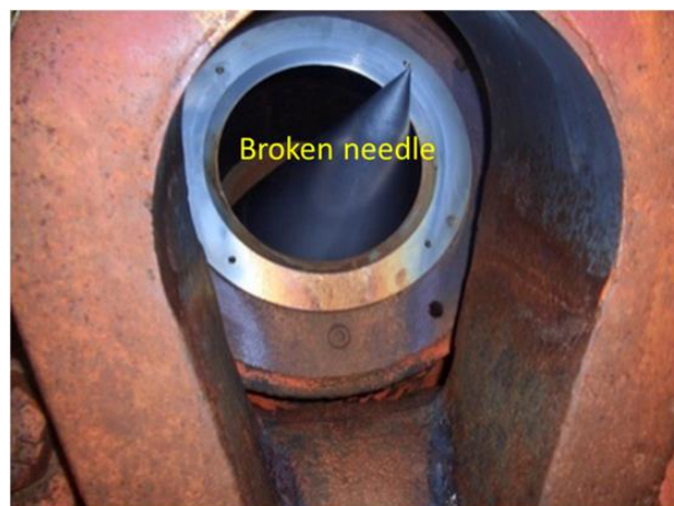
Figure 6.12. Injector damage in Pelton turbine
