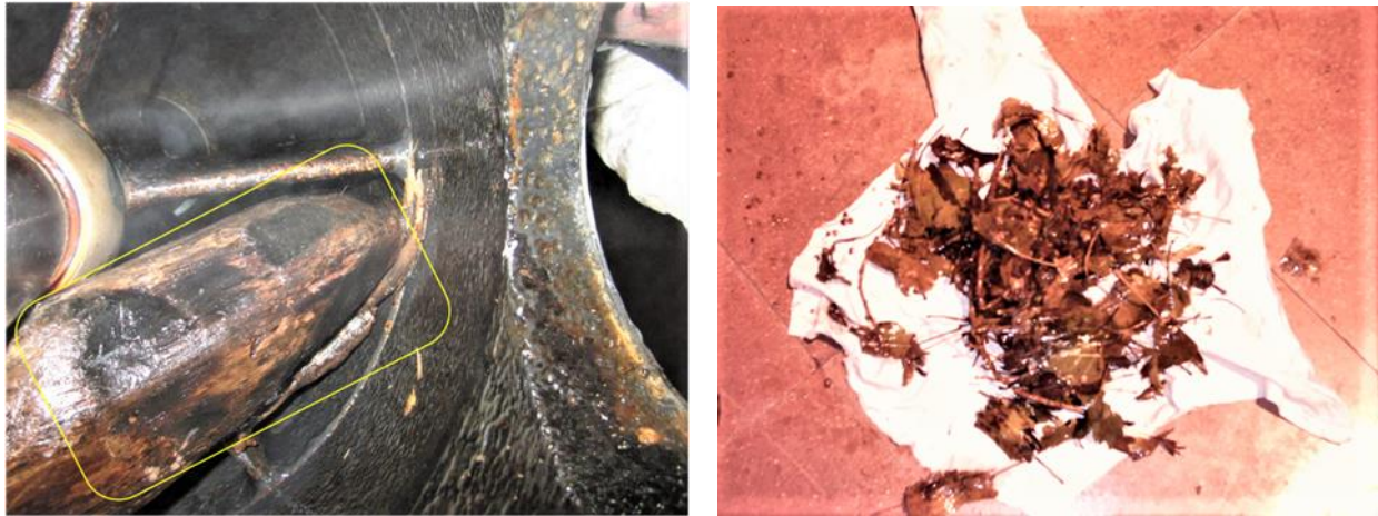
Figure 6.13. Examples of blockage in Pelton turbine injectors
