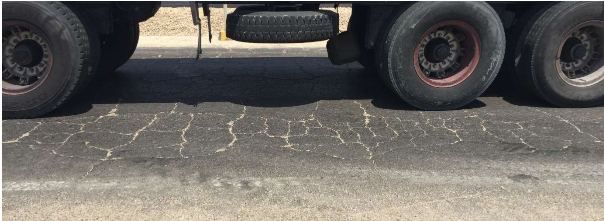
Figure 4- 4: Cracks of the old road
