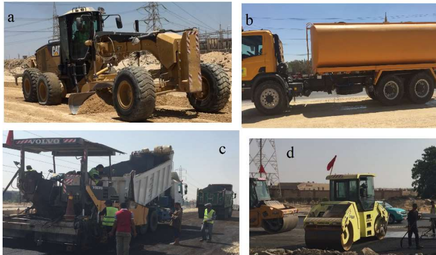
Figure 4- 5: Road project machines: (a) Grader, (b) Water sprinkler, (c) Paving finisher and (d) Double Drum Roller
