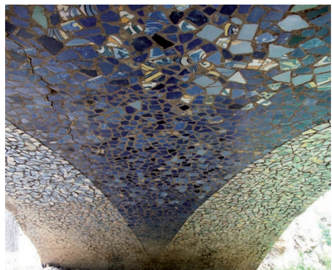
Fig. 21. Bottom surface of the Cova Cascada bridge; it can only be seen reflected in the water (1907).
