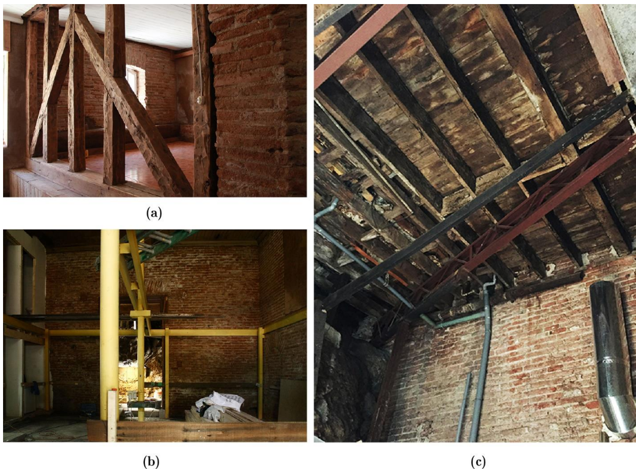
Figure 4-15. Typical features of masonry buildings in Valparaíso: (a) timber frame internal partition in Urriola street, (b) steel reinforcing structure, (c) timber story with reinforcing steel truss in Almirante Montt street.
