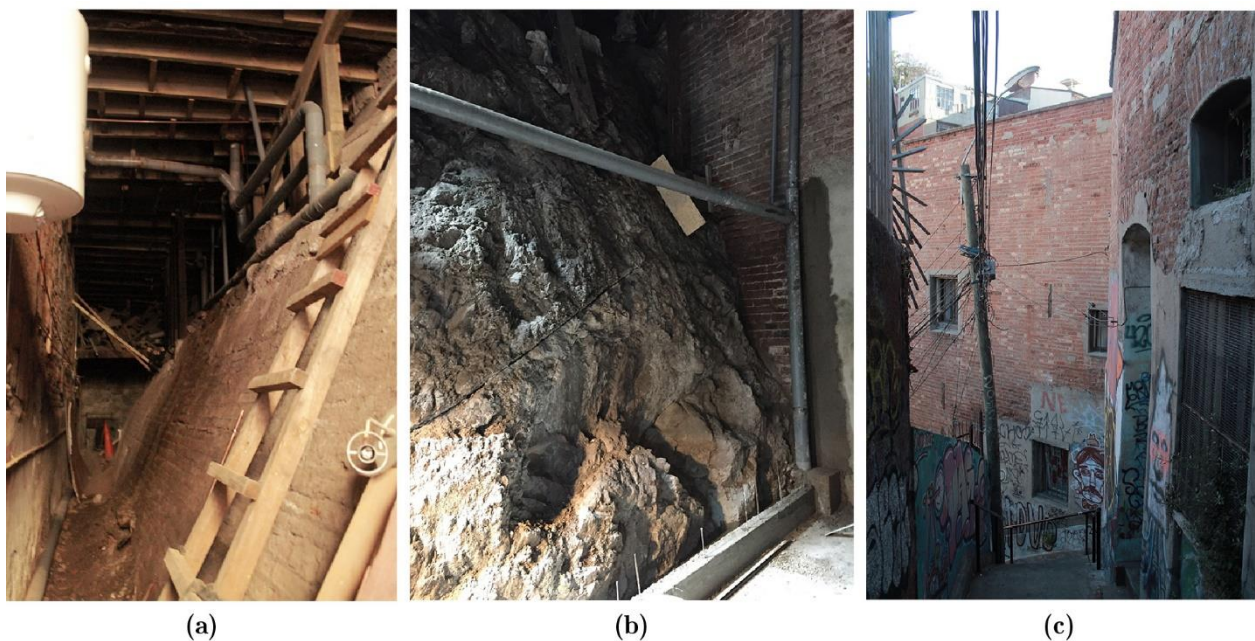
Figure 4-16. Typical features of masonry buildings in Valparaíso: (d) gravity wall, (e) rock hillside visible from the interior of a building, and (f) side wall.
