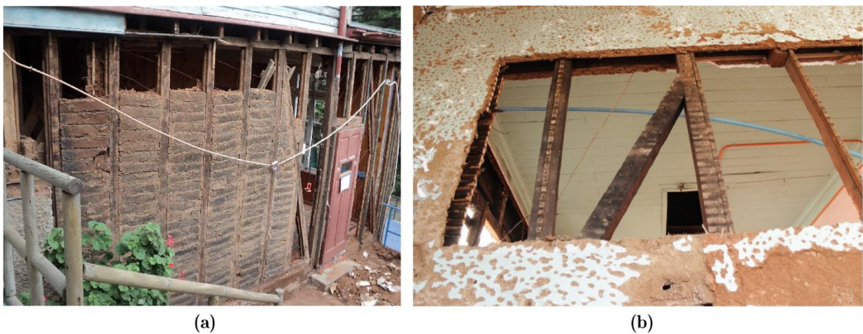
Figure 3-25. External wall filled with adobe blocks and (b) internal wall covered using the lath-and-plaster technique.
