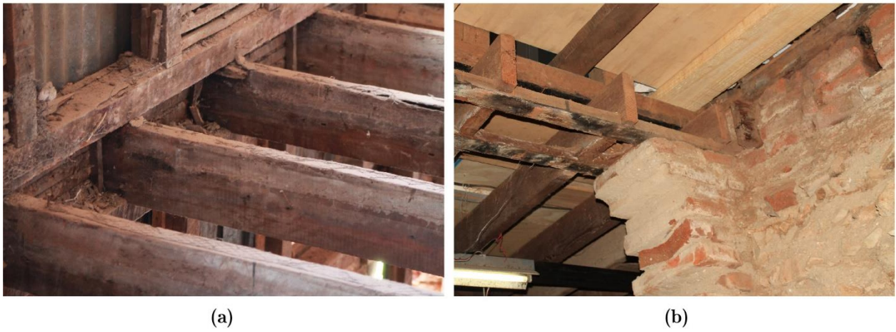
Figure 6-10. Storey system configurations: (a) joists between top and bottom sills of the walls and, (b) joists embedded into the masonry strip footings.
