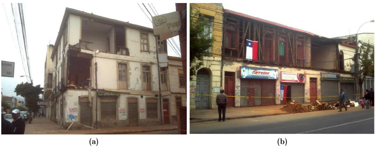
Figure 3-9. Timber frame buildings damaged after the 2010 earthquake in the down town area of Valparaíso: (a-b) partial overturning of the façades. (Photos by Lautaro Triviño)
