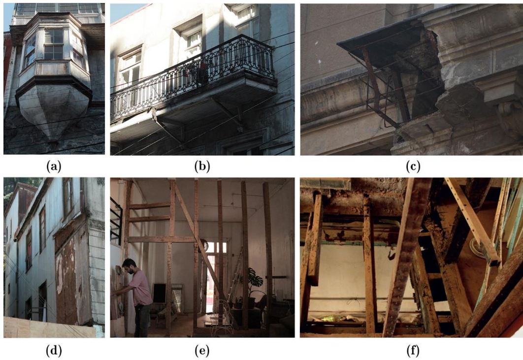
Figure 4-28. Representative non-structural elements and damage conditions: (a) large dimension bow-window, (b) poorly connected balcony, (c) severe damage of RC cornice, (d) sheathing detachment, (e) empty timber frame wall and (f) timber joists attacked by termites.
