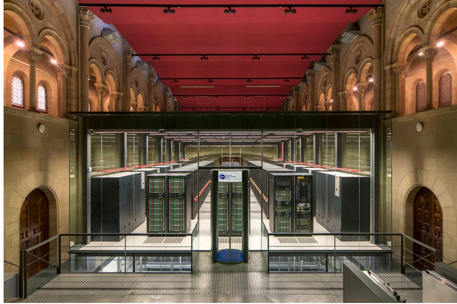
Figure 1.3: MareNostrum Supercomputer, located in an old chapel in the Barcelona Supercomputing Center. BSC.
