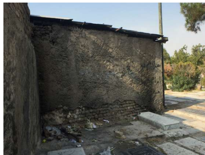
Fig.115: Environmental damages inside the cemetery, 2019
