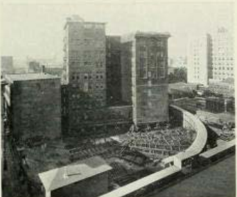
FIGURE 12. November 8. The rear of the building begins to show in this picture.
