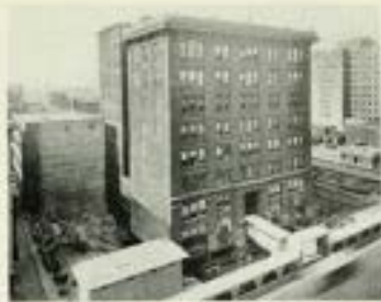
FIGURE 5. On October 18 the structure had reached the end of the straight move.
