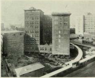
FIGURE 10. November 4. The front face of the building has now disappeared from view.
