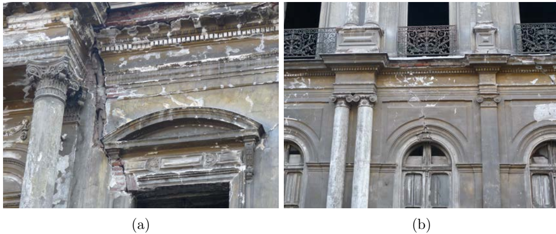
Figure 7.14: South facade Palacio Pereira: Photos of damages present in the facade after the 2010 Santiago de Chile earthquake, showing large shear cracks in and above the spandrels of the window openings
