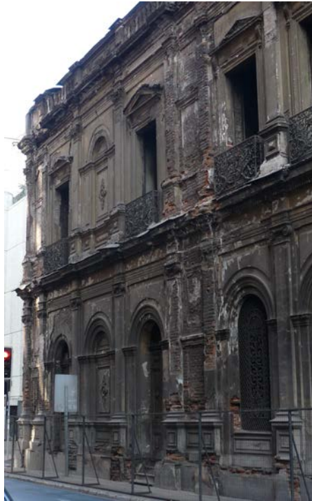
Figure 7.18: Photo of damages in the Palacio Pereira east facade after the 2010 Santiago de Chile earthquake, showing shear cracks over the openings at the most southern part of the facade
