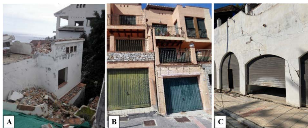
Figure 32 Examples of landslide-field evidences and damages in Cerro Gordo. Image A belong to class 6 (partial collapses), Image B is an example of class 5, a very serious damage, with a distinct crack (separating two blocks) and tilts affecting the garages. Images C shows an example of wall cracks belonging to class 4 (serious damage).
