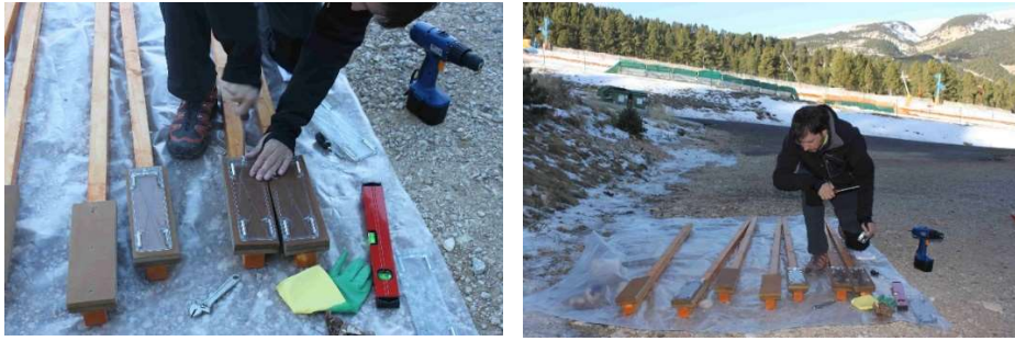
Figure 2. 25 Images of the pre-assembly of rain gauge masts, in Port del Comte (December 2013)
