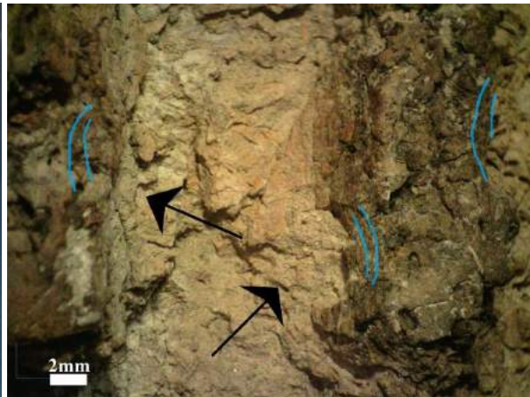
Fig. 2 Internal Surface, humps
