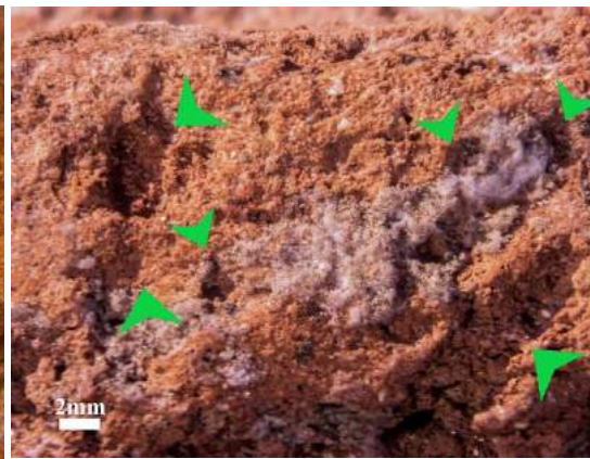
Fig. 4 Internal surface, high point
