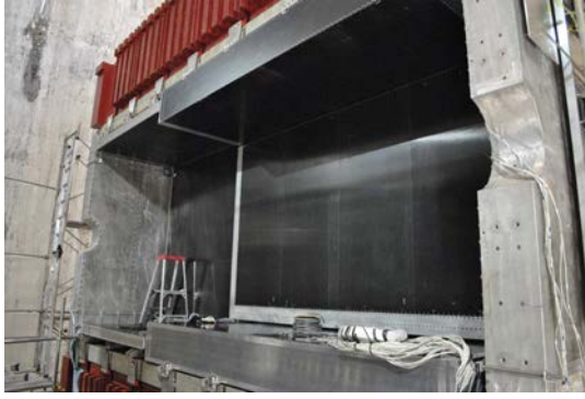
FIGURE 5.21: Picture from the original installation of the ECal in ND280. In the image, half of the ECal can be seen with the three PØDE-Cal modules on the left, and the three BarrelE-Cal modules on the right. Part of the magnet yoke (top, red) is visible. Figure from Ref. [449].
