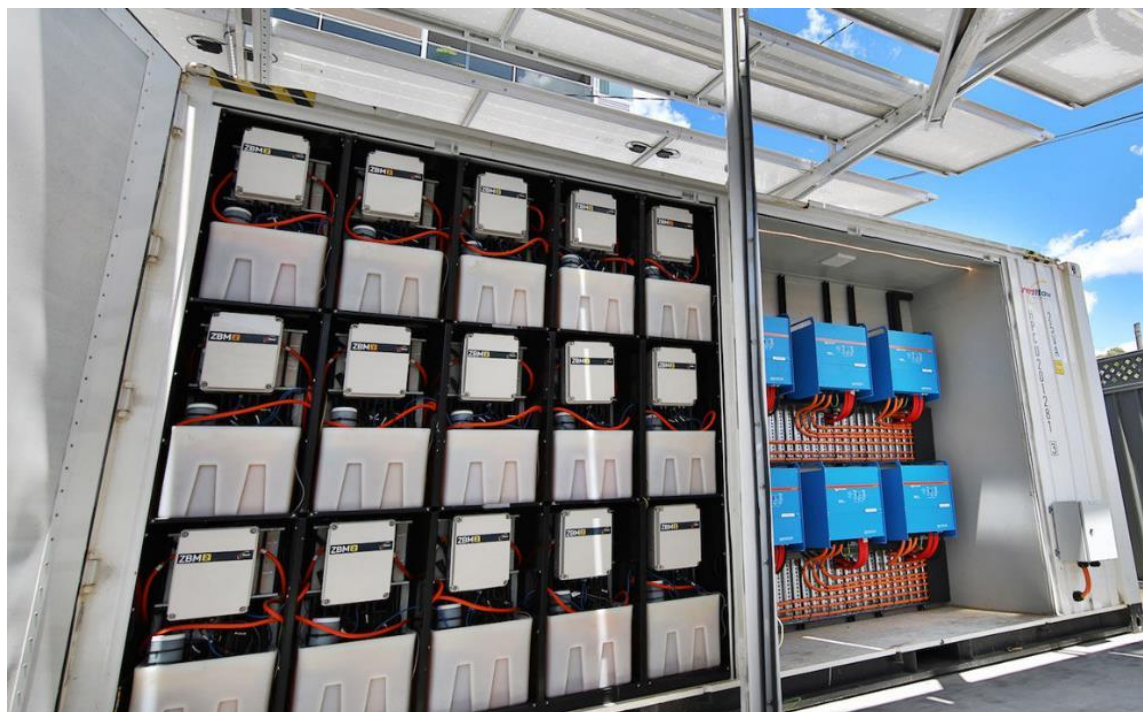
Figure J.2. Typical flow battery installation showing three rows of stacked cells. Photo credit: Redflow Limited
