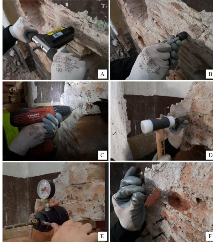
Fig. 49 Minor Destructive Technique (MDT) steps executed in existing masonry buildings. A) The PPT device positioned perpendicularly to the surface to be tested, B) the micrometre inserted to the hole to read the penetration produced by the PPT device, C) the rotary-hammer drill used to make the HPT pilot holes, D) the helical tie of the HPT hammered into the pilot hole, E) the HPT grip lever applying the load by turning it manually until failure, F) the failure mechanism in brick specimens testing the HPT
