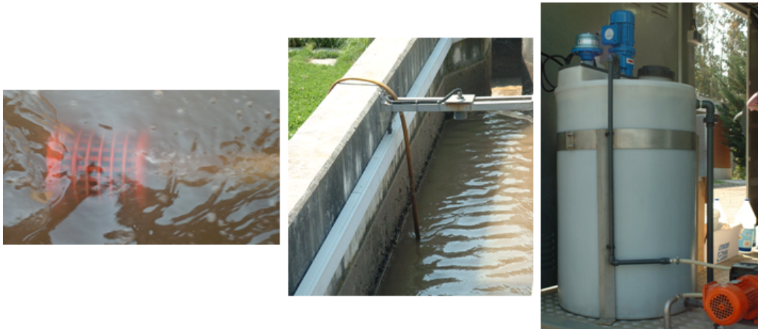
Figure 2.5: Storage tank Filling
