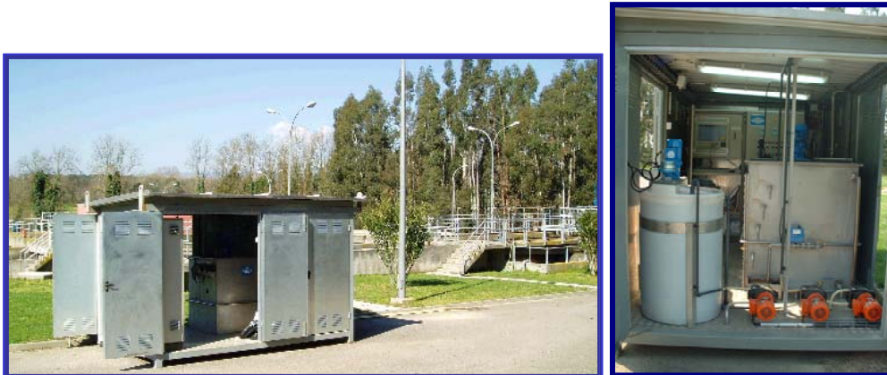
Figure 3.3. Picture from outside and inside of the SBR pilot plant.
